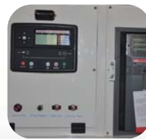
Control Panel & MCB
